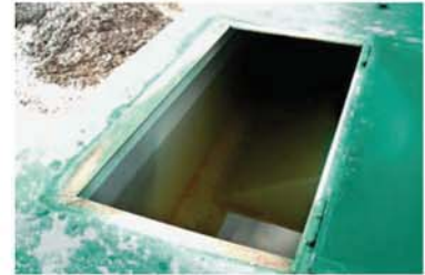
Separate cabinet area stores liquids to be pumped out.
