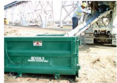
Watertight container minimizes the risk of caustic wastewater being disposed improperly.
